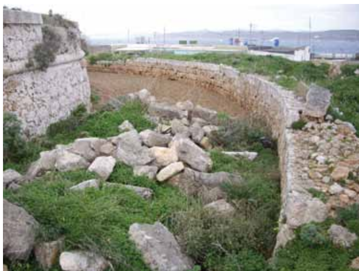
Makeshift field and collapsed masonry in the ditch of Ta' Mačċu Battery
