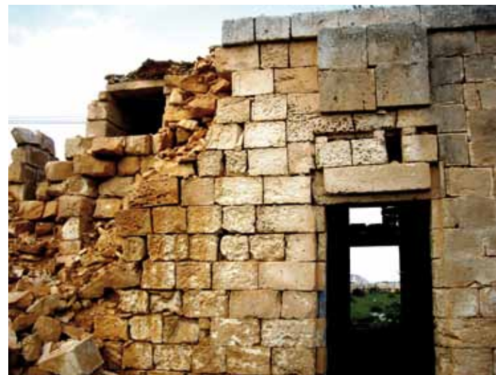
Crivelli battery falling apart
