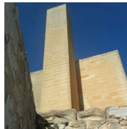
The boiler chimney acting as a discreet vertical element, perhaps inspired by a village church steeple that crowns the old barrack complex (Photograph by Nicholas Farrugia)
