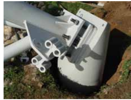
Complex foundation detail to receive various tension connectors, and to adjust position of contact between arch and ground
