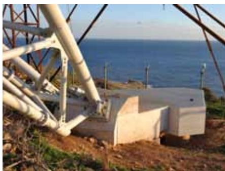
Foundation designed to transfer arch support point to area where piles could be driven into rock
