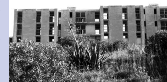
White Rocks complex - gutted but still standing strong (Photograph by Nicholas Farrugia)
