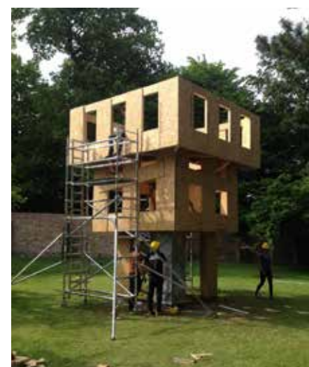
Zinc cladding taking place once the substrate structure was complete (Pavilion construction)
